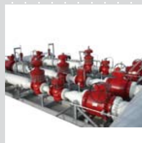
Pressure reducing stations
